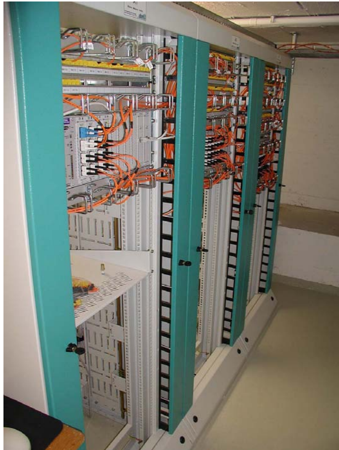
Figure 16: In the basement of the WMI a new stacked switch providing 68 fiber optic connectors was installed to switch data packets within the WMI as well as from the WMI to the internet and vice versa.
